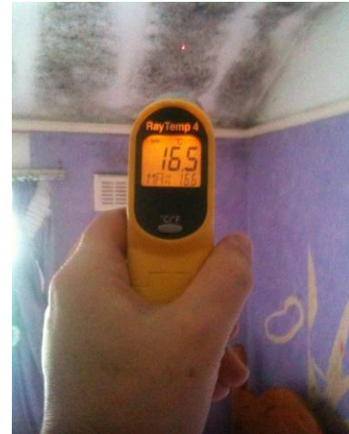
The gap between the roof and ceiling was omitted
