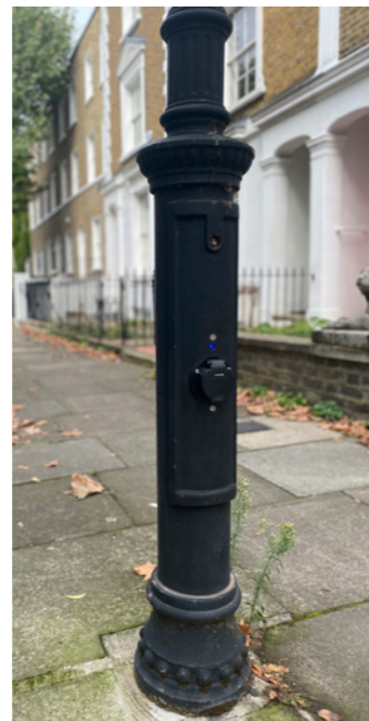
◀ A lamppost charger on a residential street.
