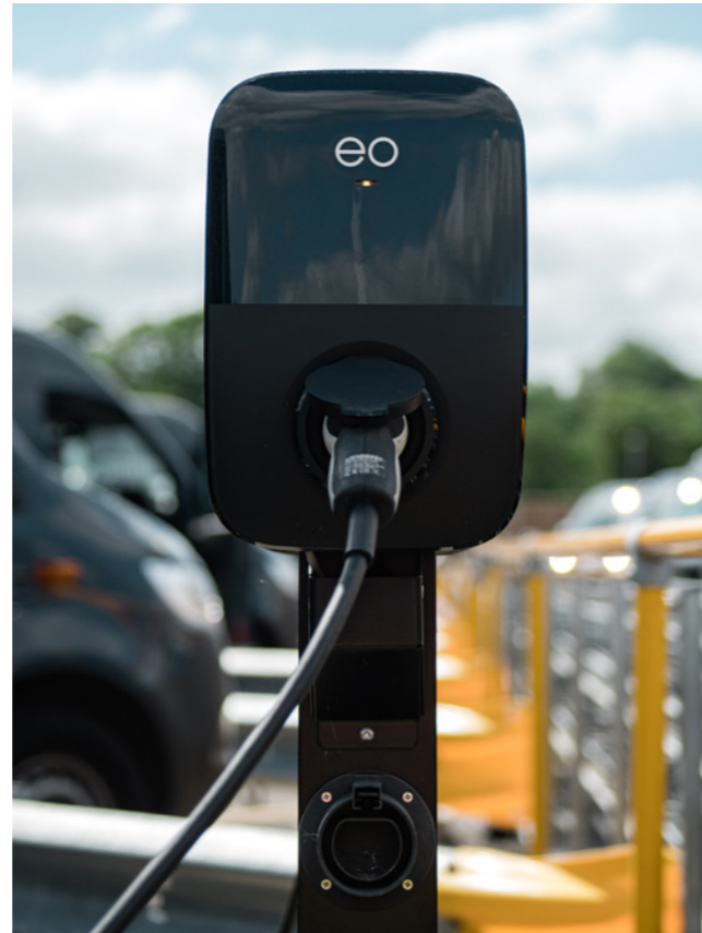
Charging solution at a van depot.
