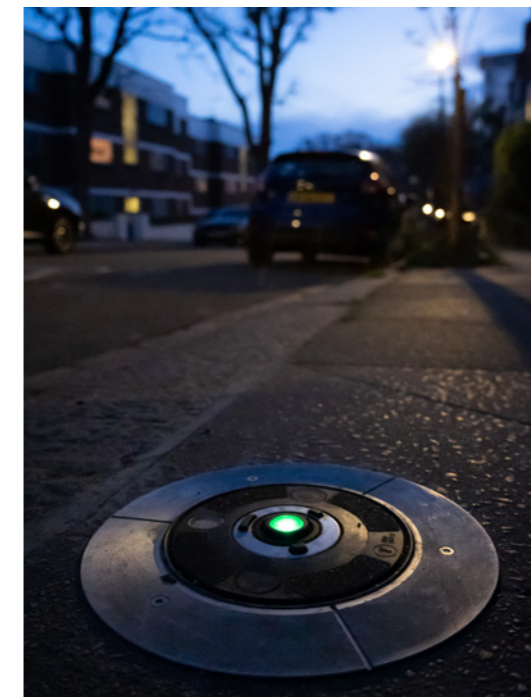
Private on-street AC charging solution. Shown hidden.
