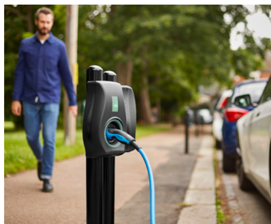
◀ A chargepoint on a residential street.
