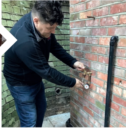
02 Undertake a water pressure test to prevent damage/failure to the softener unit as a result of too lower/higher water pressure
