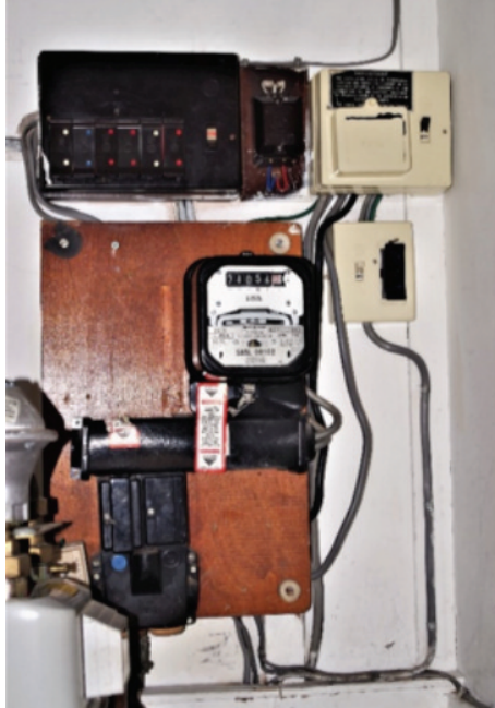
FIGURE 1: MAINS PROTECTION AND METERING IN OLD RESIDENTIAL BUILDING
